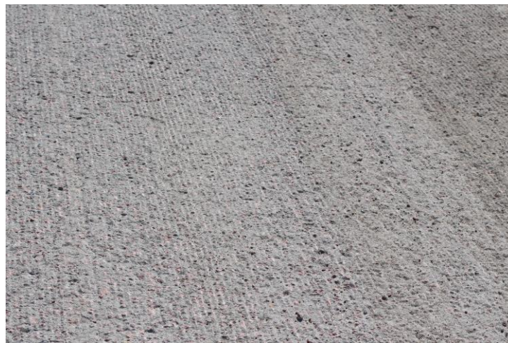
Figure 3-11. Photo of substrate surface conditions of site E3
