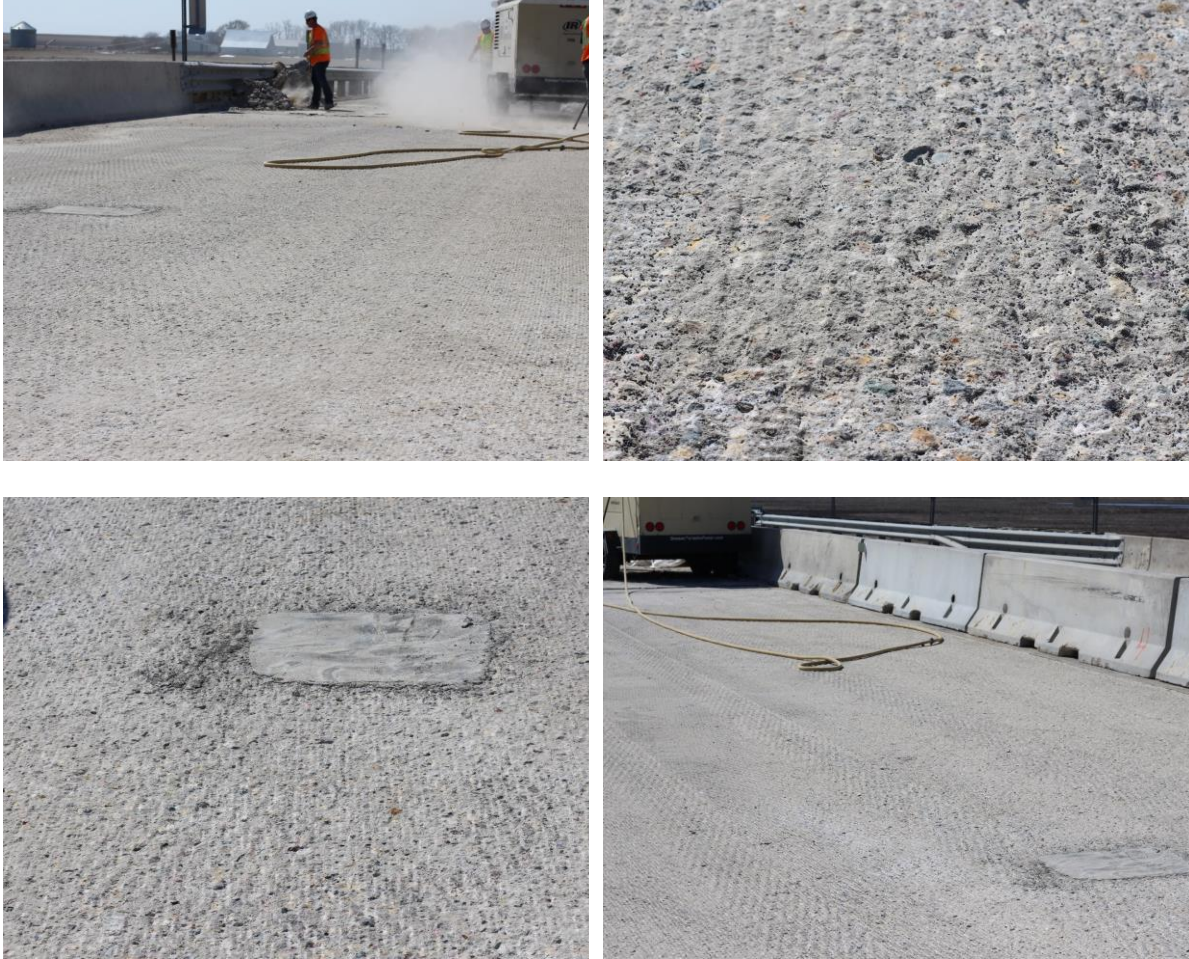
Figure 0-4. Surface condition of bridge deck of site E1 prior to overlay
