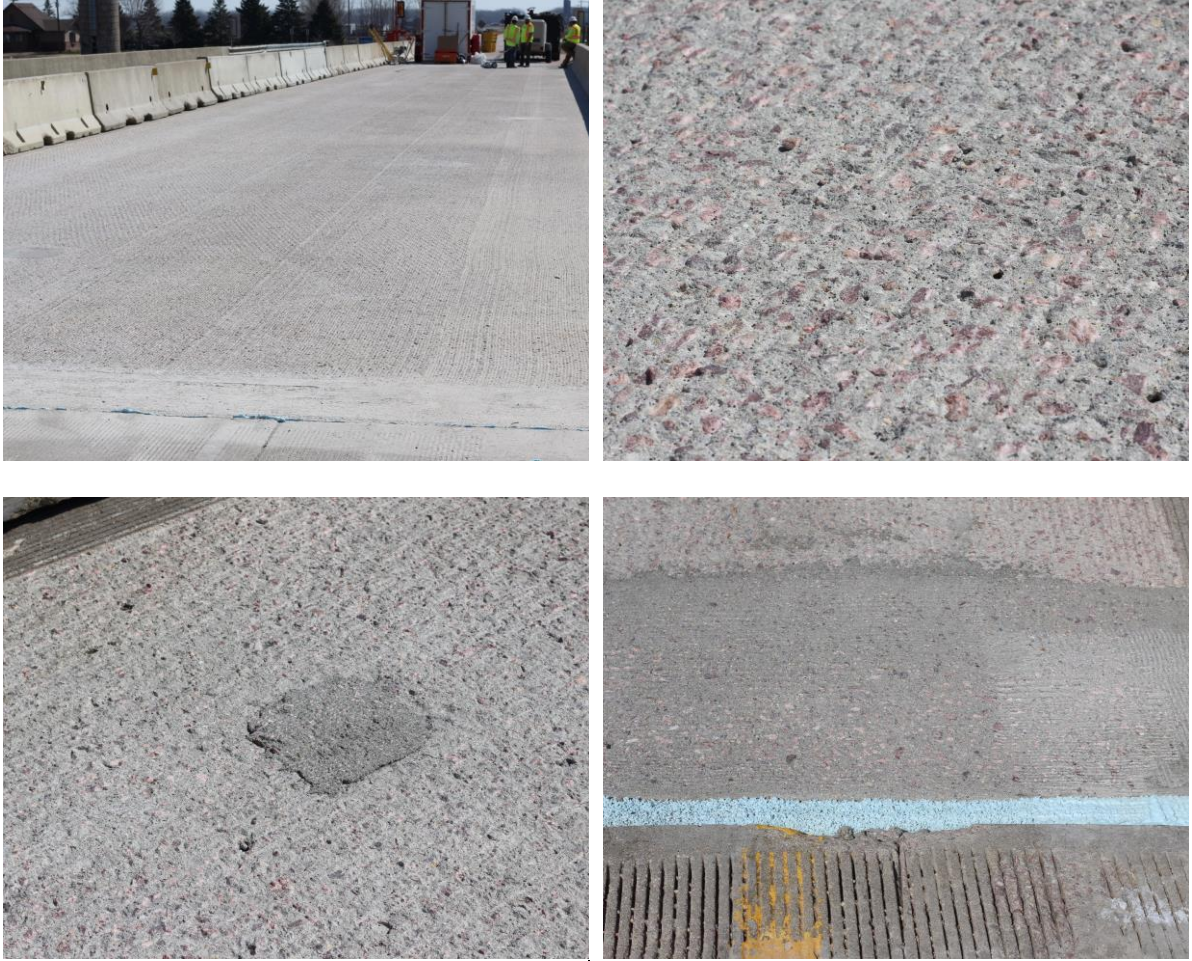
Figure 0-5. Surface condition of bridge deck of site E3 prior to overlay
